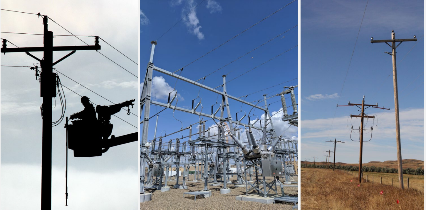
McKenzie Electric Cooperative left photo: a picture of one a linemen during a pole changeout; middle photo: The inside of the substation at the ONEOK Demicks Lake substation; right photo: copper line replacement. McKenzie staff keep busy serving, focused on affordable, reliable electric service to their member-owners.
