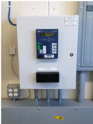
Chapman Metering installation
