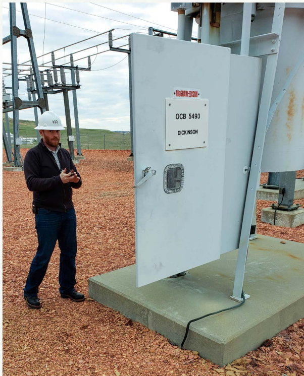
Eric Boesse-HDR joined Jeremy Mahowald and Gary Markwart – MDU on the annual facility inspection.
