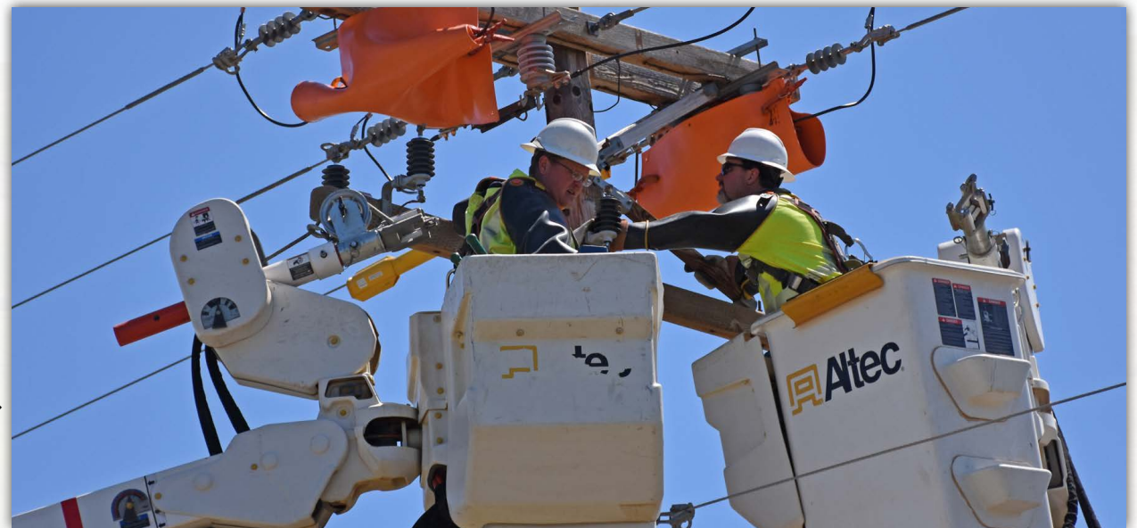
In May 2019, Roughrider Electric Cooperative crews cut in → bypass switches and installed new Versa-Tech breakers. This crew included Linemen Brock Swensrud (left bucket) and Dion Gefre (right bucket). Photo Credit Roughrider.
