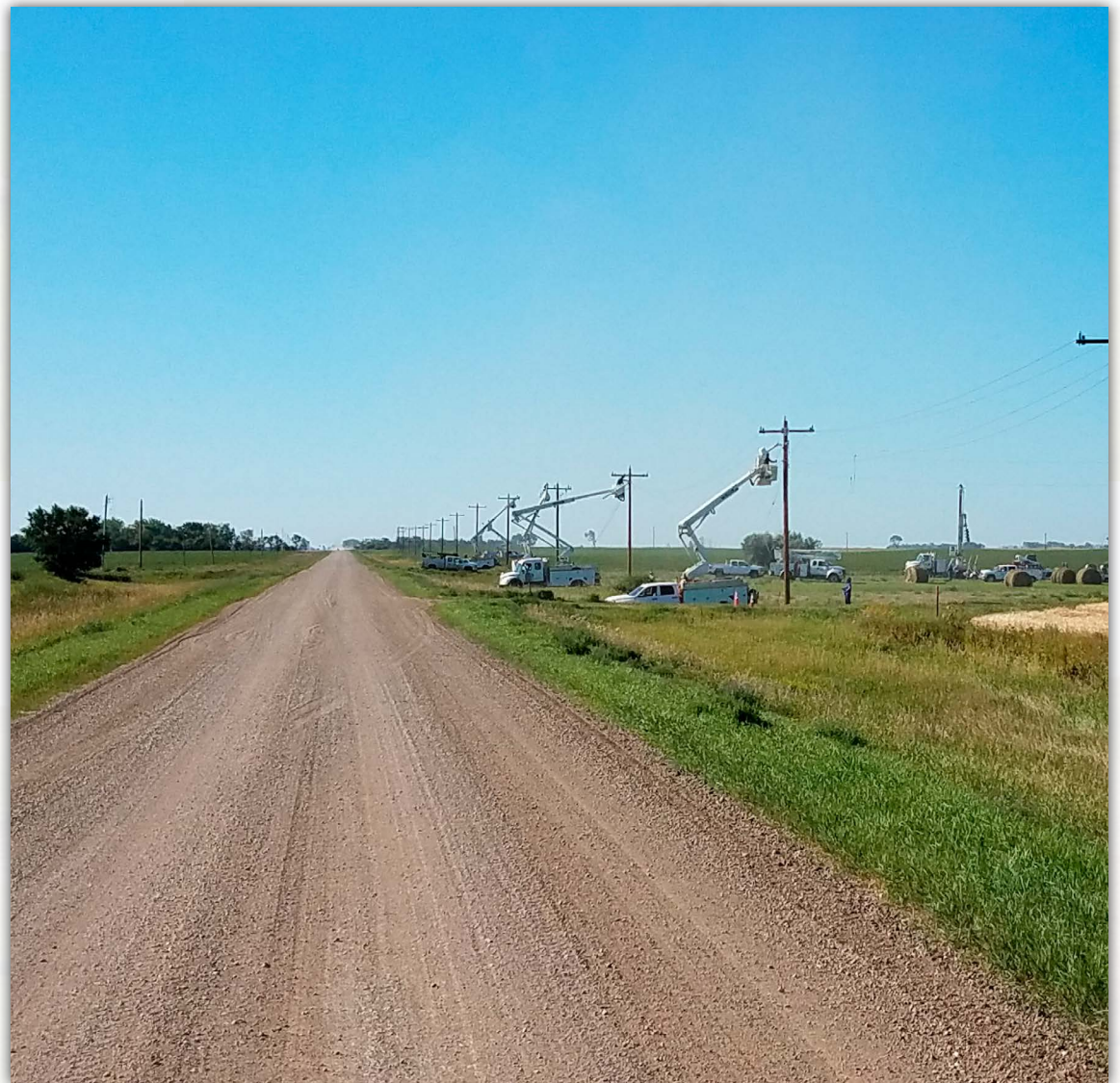
2019 marked the completion of the largest construction workplan in the history of Burke-Divide Electric Cooperative . $27 million was invested in the Cooperative's infrastructure over a period of four years. The plan focused on system reliability and included projects such as construction of new lines, upgrades to existing lines, and installation of updated meter technology.
