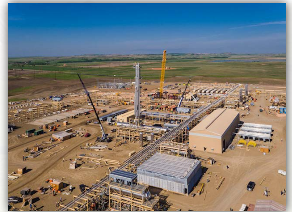
McKenzie Electric Cooperative's Demicks Lake Substation built in 2019 to serve oil and gas development.
