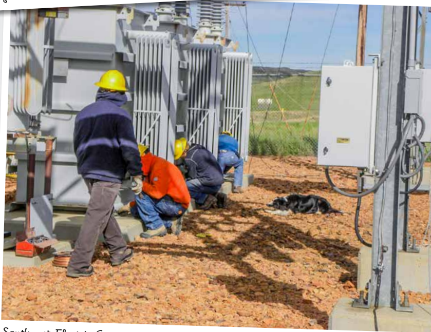
Southeast Electric Cooperative has done much needed updates on two of their substations this year. Under the supervision of "Bo," the linemen are removing bolts from the transformers so the crane could lift them out of the Willard Substation.
