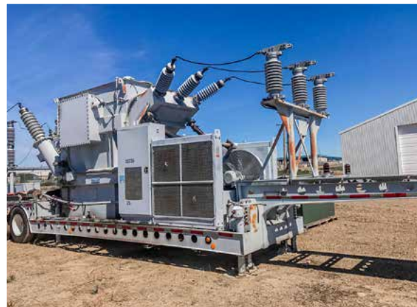
Upper Missouri/MorGranSou/MDU shared mobile transformer ready for transport to Jordan MN
