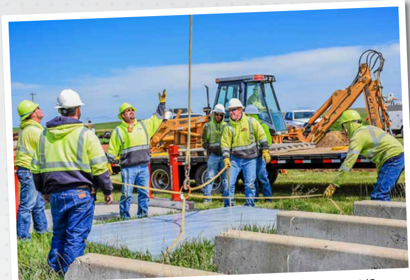
Slope Electric Cooperative hosted trench box safety training in May 2017 in a pole yard near New England headquarters. More than 25 employees from Slope, Roughrider Electric Cooperative, 3C Construction and Innovative Energy Alliance Cooperative attended and learned how to assemble an aluminum box, that when lowered into the ground, will protect the worker from injury if the dirt wall collapses and fills the hole.
