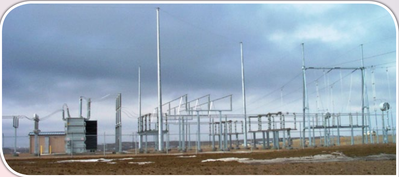
Little Missouri Substation
